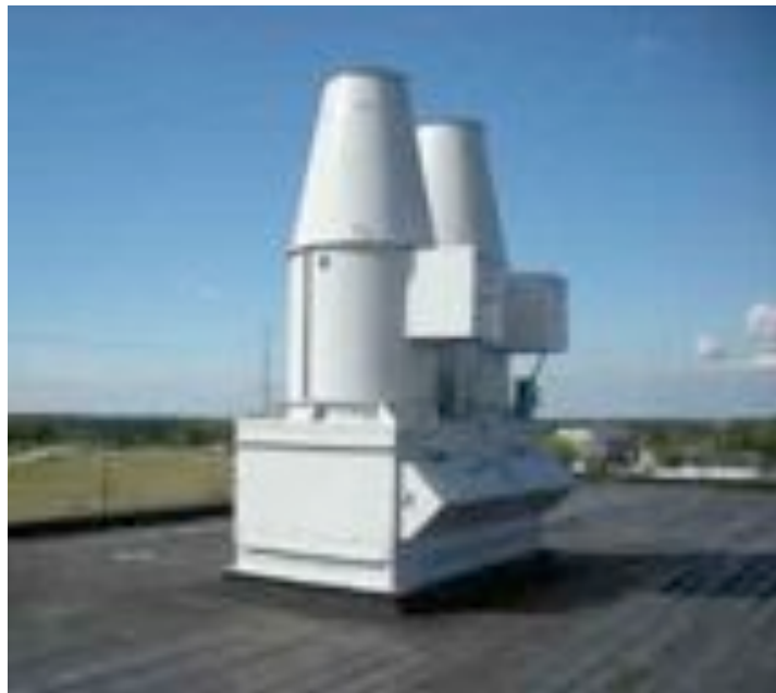
CLEAR THE AIR State-of-the-art exhaust fans are one component of a sophisticated HVAC system designed for maximum sterility.
