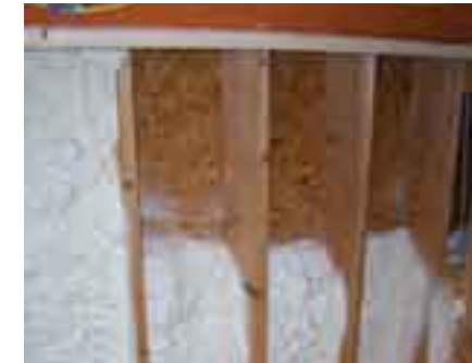
JOB APPLICATION Icynene foam insulation can be spray applied or “poured” into wall cavities.
