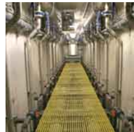
CLEAN LOOK CT Consultants provided its services at McFarland Creek Wastewater Treatment Plant.
