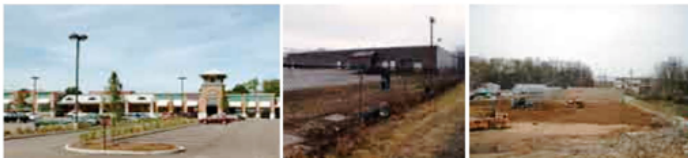
STAGING A SOLUTION The Middlebury Marketplace site (left) required significant cleanup (center). As part of the redevelopment process, a four-foot "clay cover" was utilized to protect occupants of the building (right).
