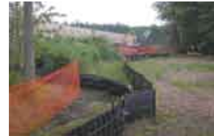
BUILDING A BARRIER A silt fence was installed along the perimeter of the Lighthouse Village retail development to reduce the amount of sediment flowing into nearby wetlands.
