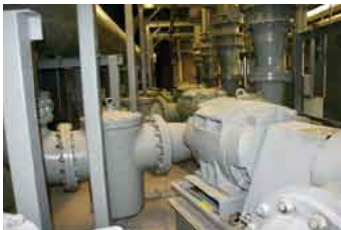
BIG BACK-UP The central chiller plant is capable of producing approximately 3,300 tons of cooling when operated under emergency back-up power.
