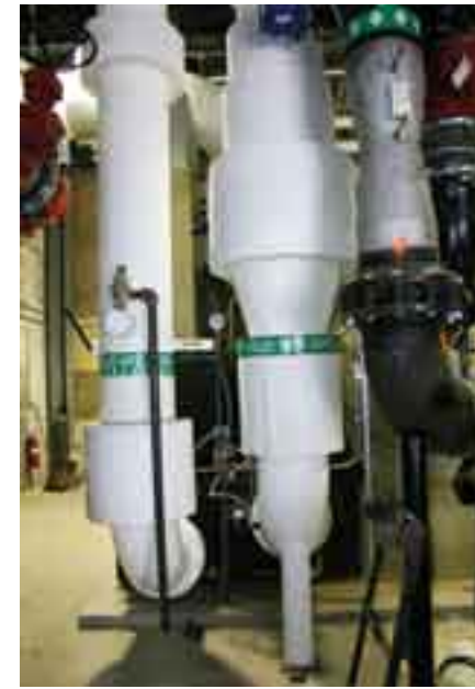
AIR FOR THE AREA The power plant, which is presently being brought online, supports air conditioning, cooling and dehumidifying for the entire Cleveland Clinic campus.
