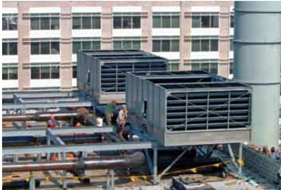
TOWER OF POWER Chiller heat is rejected to a roof-mounted cooling tower farm consisting of two four-cell, crossflow axial fan cooling towers with each cooling tower capable of 4,400 tons.
