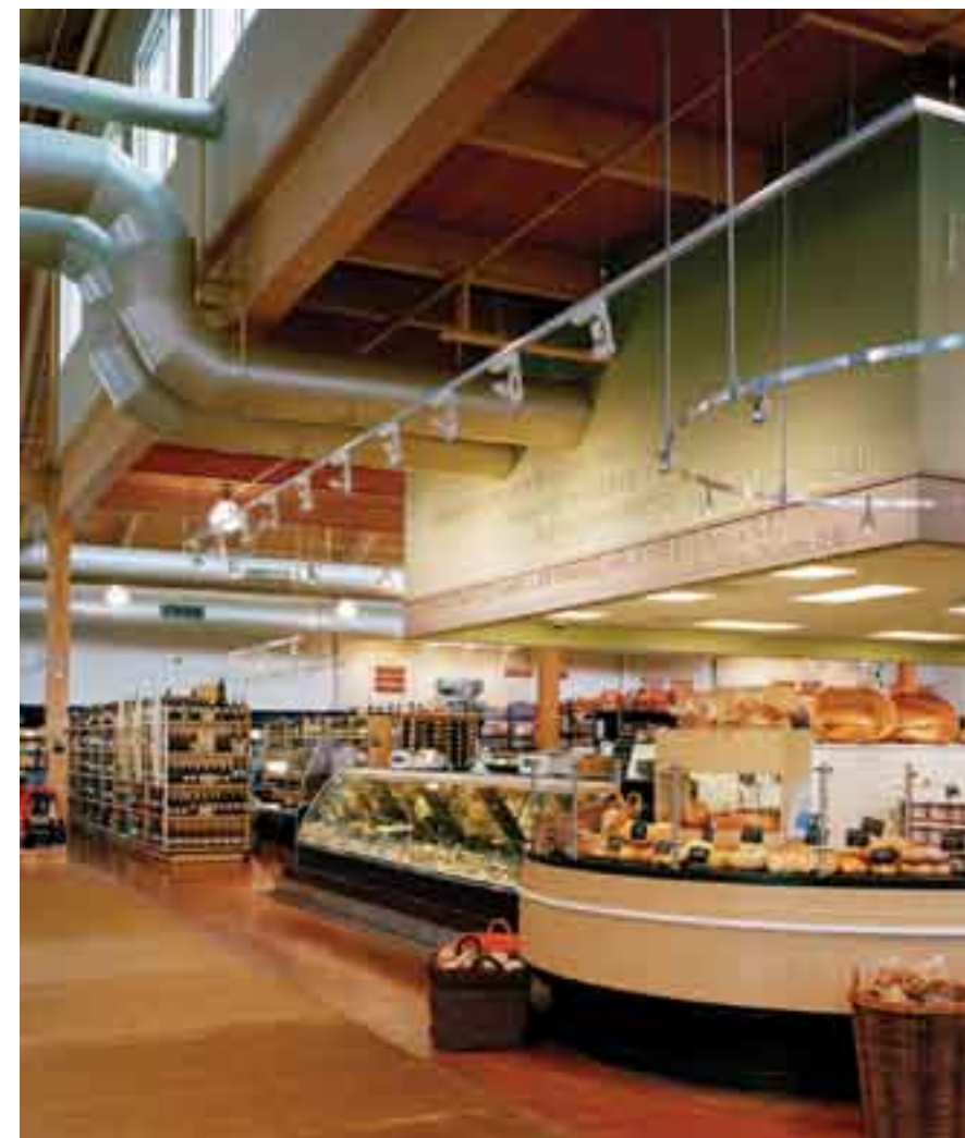
OPEN AIR Exposed, round, champagne-colored supply ducts extend over much of the ceiling and fit right in with the historic design.
