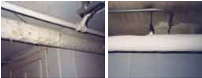
CLEAN COVER A problem area (left) has been corrected with preventive measure encapsulation (right), which is an efficient alternative to asbestos removal when possible.
