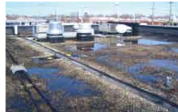
SAFE COVER At the Snow Road Plaza in Parma, the newly installed four-ply tar & gravel built up roofing system can still pond water, but tar's inherent resistance to ponded water should provide a service life of 40 years or more.
