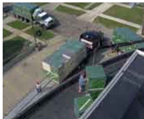
TOP SHAPE Absolute Exteriors completes work on the natatorium's new tapered roof.
