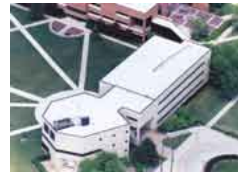
WEATHER PERMITTING The Duro-Last roofing system installed at Terra Community College in Fremont, Ohio was selected in part because of its ability to withstand high winds.
