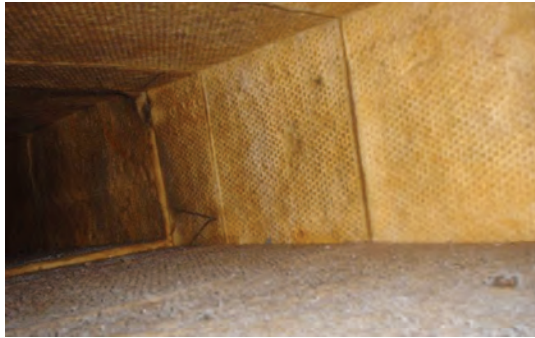
WASTED WORK Damage to fiberboard ducts during cleaning procedures can result in fiberglass dispersion and increased complaints.
