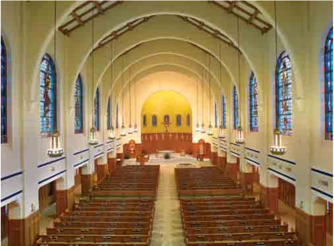
ROW BY ROW As part of the renovation, all of the solid oak pews and kneelers were carefully removed, transported to Henniger's workshop and then stripped and artfully refinished.
