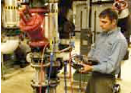
Photo courtesy of Kahoe Air Balance Company
