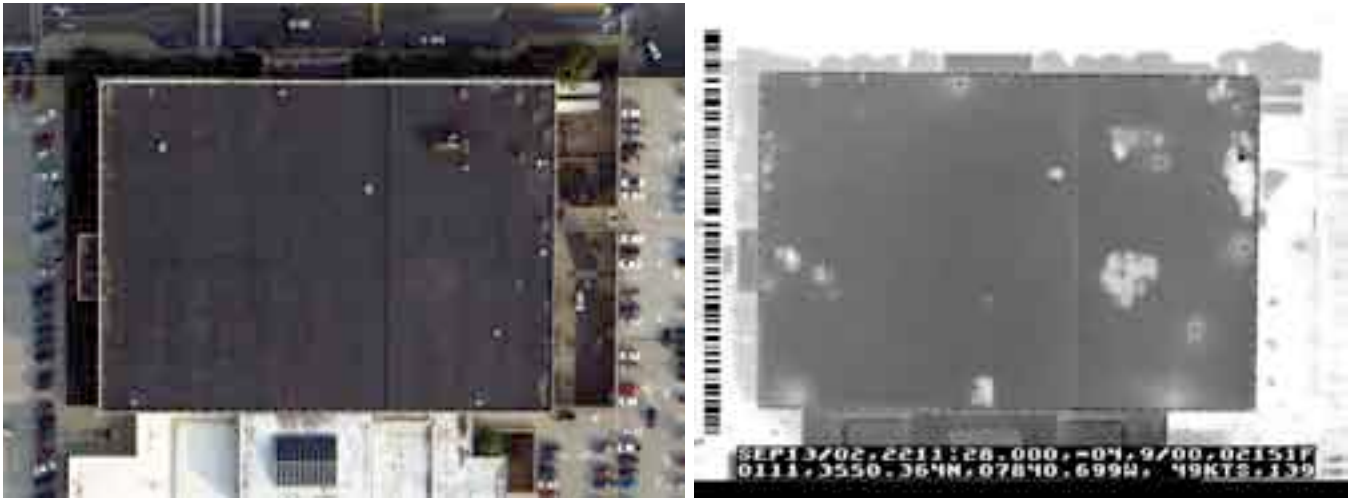
TWO VIEWS Infrared imaging (right) can reveal problem spots on roofs not normally visible to the naked eye (left).
