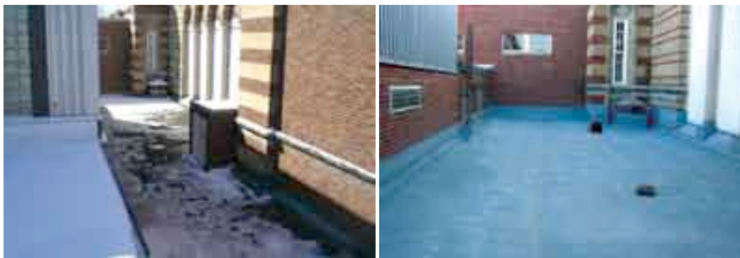
DRAMATIC DIFFERENCE LaGrange-based West Development Group supplied the new Spray Polyurethane Foam insulation system that was recently installed on 11 schools within the Berea City School District, including Berea High School shown here before (left) and after roofing work was completed (right).
