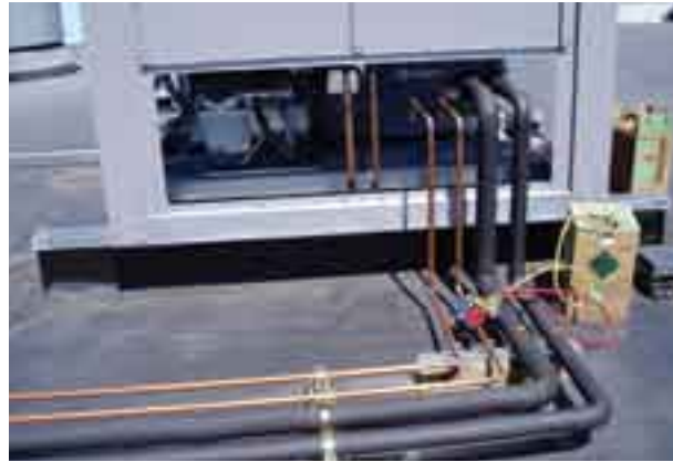
TOP SHAPE Lisco's specialties include the installation of rooftop mounted HVAC systems.
